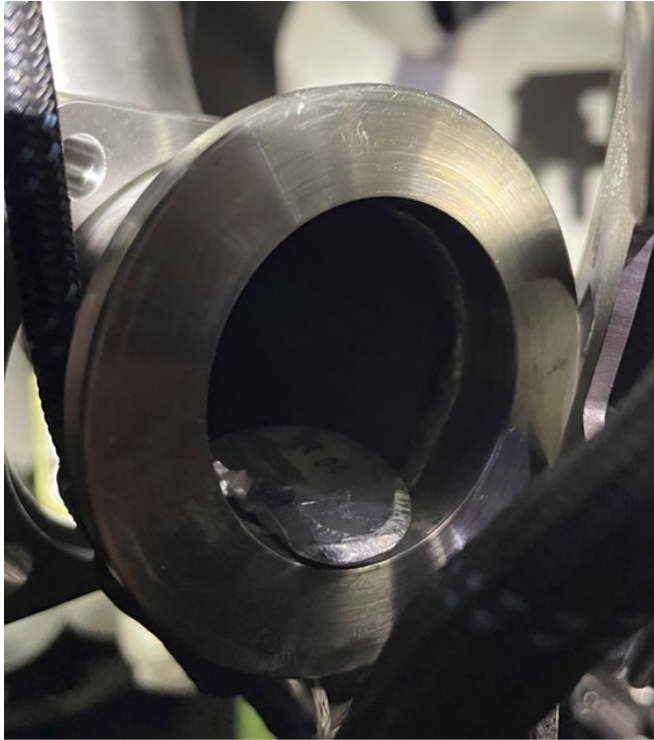
Photo 2 – Dislodged piece of check valve
