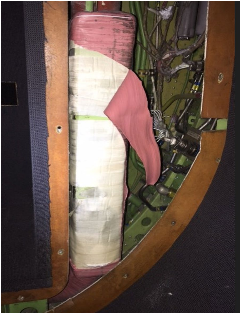
Picture 1 – Muffler as installed, adjacent to the hydraulic filter manifold, outer insulation wrapping damage is evident
