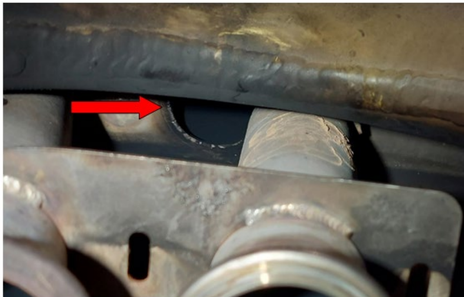
Picture 3 – Weld failure, source of exhaust gas leakage
