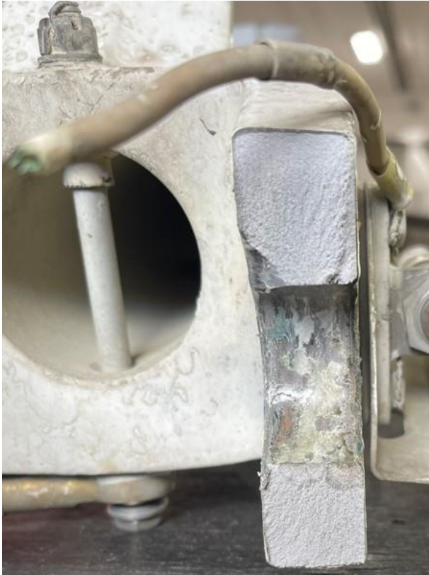
Picture 2 – Close-up of the lug with corrosion present in the bore
