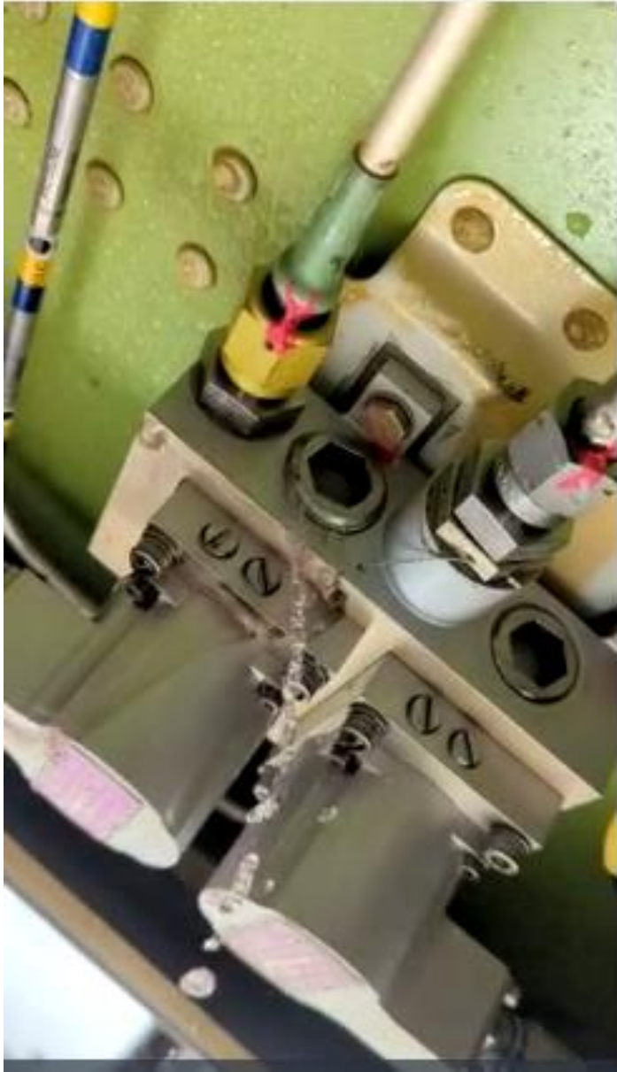
Picture 1 – Leaking Brake Control Valve
